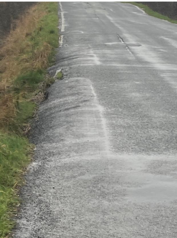
Damage to road edge.
